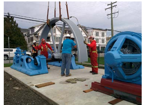
One-half of the flywheel is set in place in the Ice Machine's new location in the parking lot.
